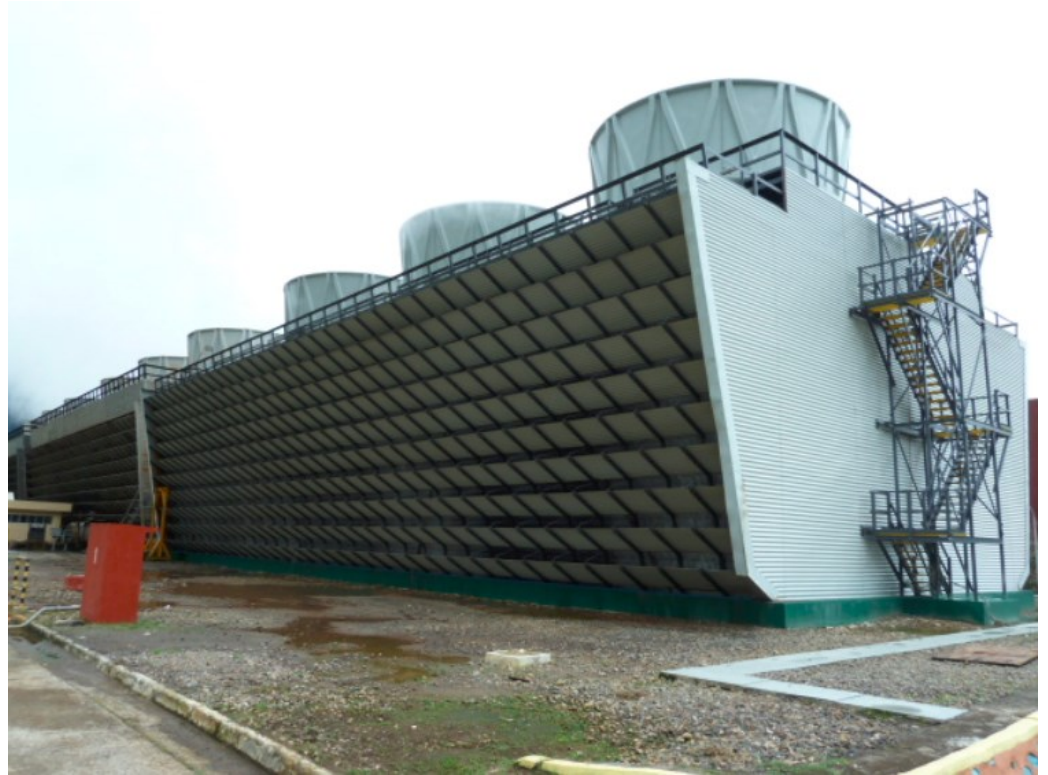
Figure 1: Cooling tower in Leyte Geothermal Production Field (LGPF).
