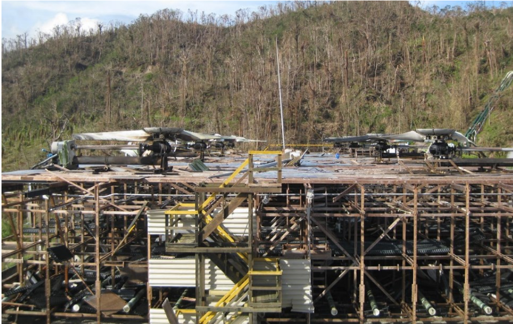
Figure 3. A damaged cooling tower in Leyte after Typhoon Yolanda.
