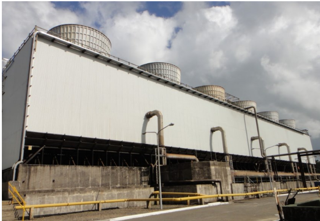
Figure 2. Typical cooling tower of EDC.
