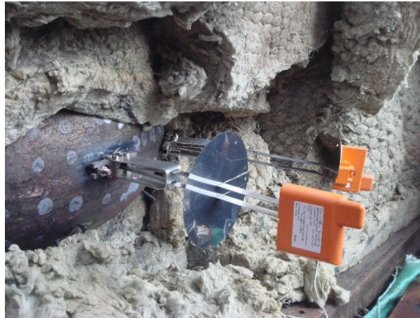
Figure 2: Carbon steel U-bend with sensor
