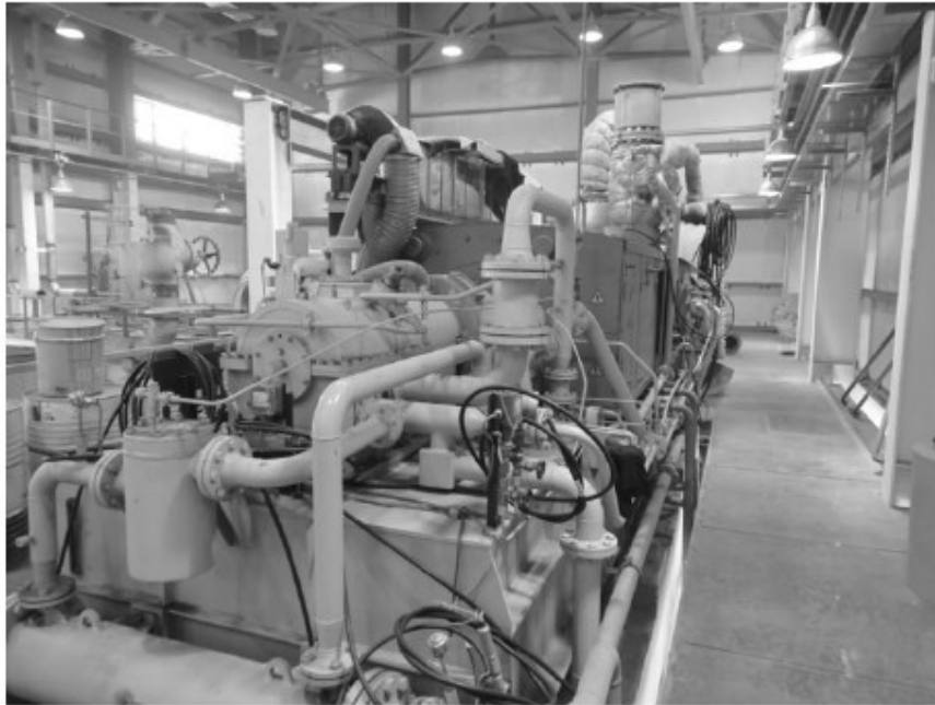
Figure 4: Pauzhetskaya GeoPP turbine unit equipped with the binary turbine produced by the Kaluga Turbine Works.
