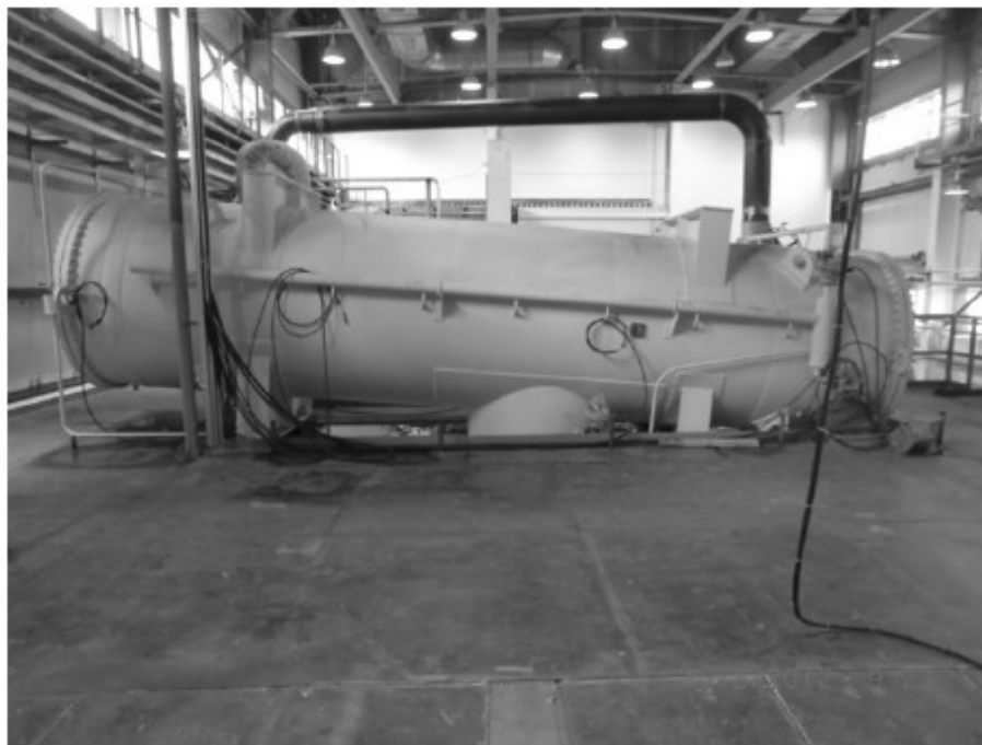
Figure 5: Condenser of the binary turbine unit at the Pauzhetskaya GeoPP.
