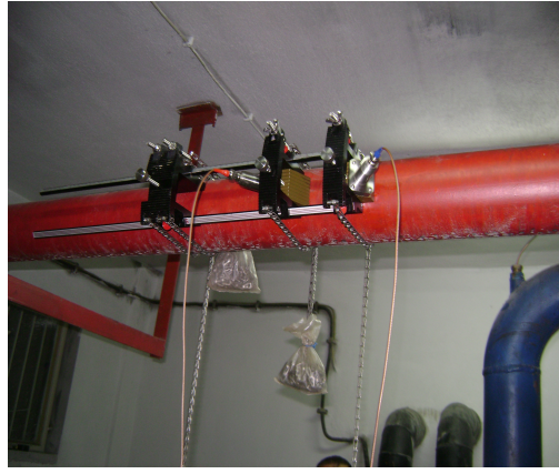
Figure 2: A view of an experimental measurement and monitoring studies on thermal water production and energy distribution pipe lines by using ultrasonic flow meter (Ozgener and Ozgener, 2009)
