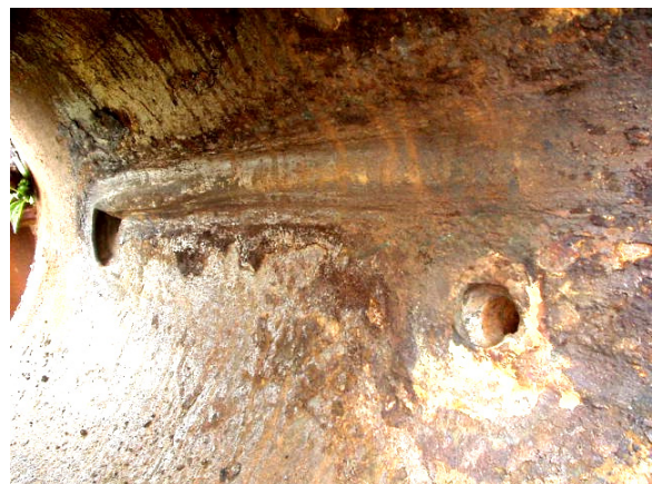
Figure 5: Damages in the tapping points of the 2-inch diameter bypass line and 1-in diameter vent viewed from inside the branchline.
