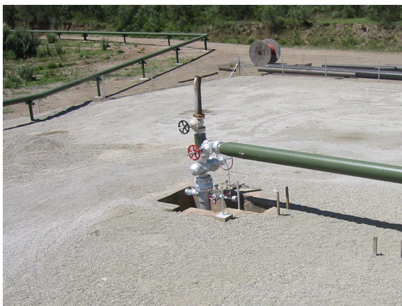
Figure 1: Well OW-202 Supplies Steam to the Oserian/GDA Turbine Generator Set
