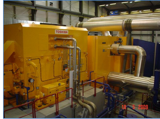
Figure 5: Turbine and generator
