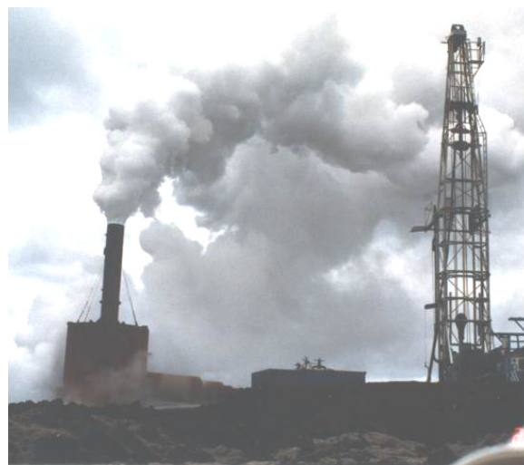
Figure 8: A vertical drum silencer with a went stack
