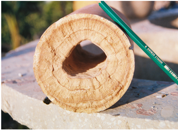
Figure 2. Thermal water pipe line scaling in Afyon Sandıklı Hüdai hot springs from hot water production well.
