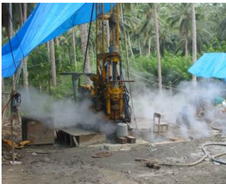
Figure 7: Flowing of hot water of the MM-1 of core in Merana field, Sulawesi-Indonesia
