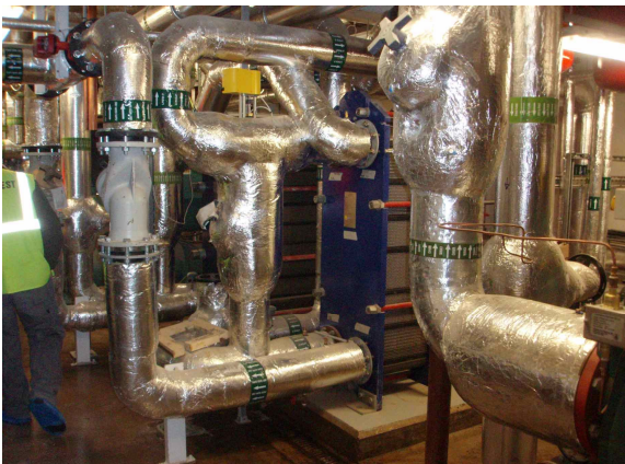
Figures 5, 6: UCC Cork IT building and plant room
