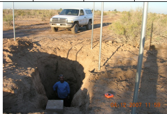
Figure 6. Preparation for crackmeter installation over the Cerro Prieto fault at F4 (Fig.1).
