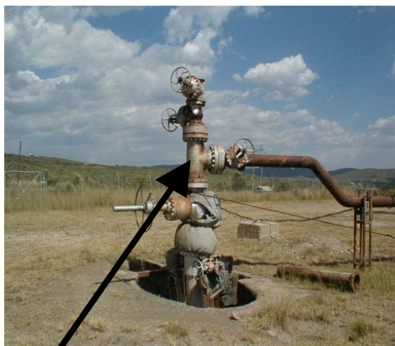
Figure 5d: T-connection on well OW-34
