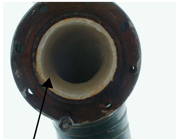
Figure 5b: Thickness of scale deposited in separated water line
