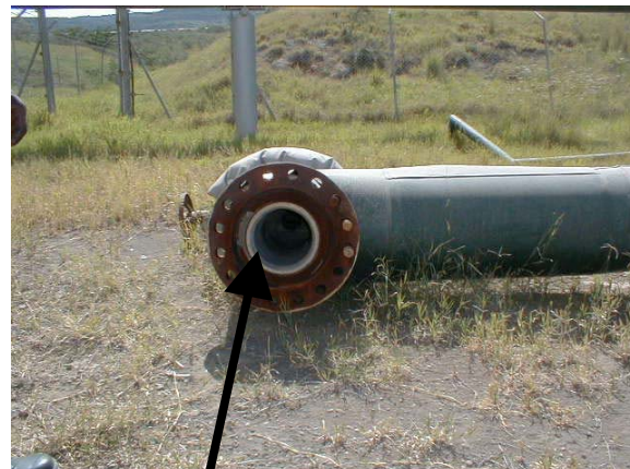
Figure 5c: Thickness of scale at the T-connection of the well OW-34
